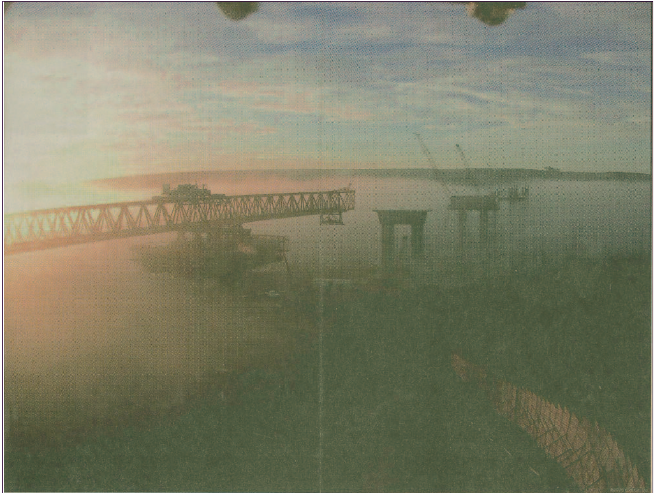
One of just two segmental bridges in California, Otay River Bridge is part of South Bay Expressway, San Diego County's first toll road. An engineering feat, once completed, the 4-lane bridge will stretch for three-quarters of a mile and reach heights of 18 stories. Photo courtesy of South Bay Expressway.
